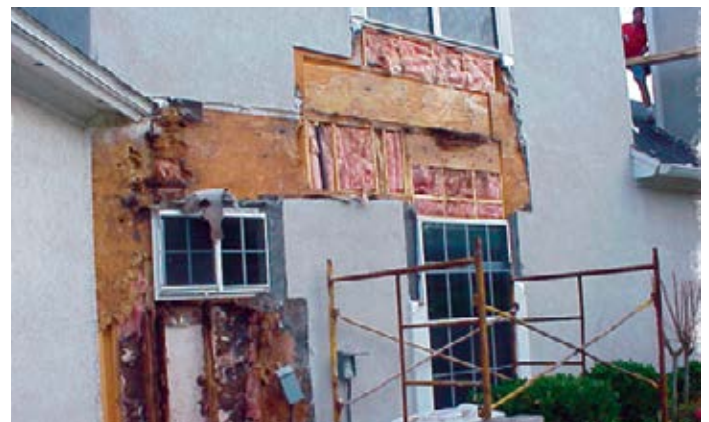
5 YEAR OLD HOME ($200K IN REMEDIATION COST)
