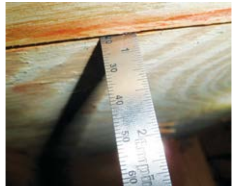
The sheathing thickness is measured. Once the inspector has these pieces of information, question 2 of the OIR-B1-1802 can be completed.
