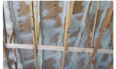
A qualifying SWR for OIR 1802 purposes. Notice the sealant is typically only along the joints.
